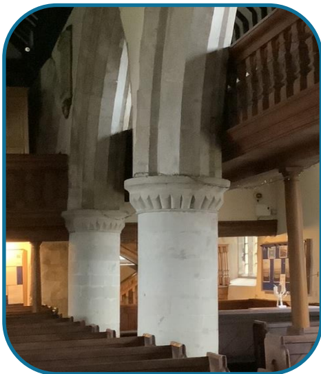
The pillars lean due to the Tudors building up the wall of the north aisle
