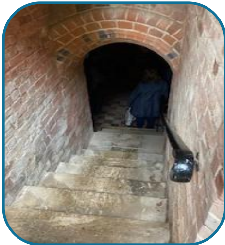
The steps into the Lovelace Mausoleum and the inside which has been restored by English Heritage
